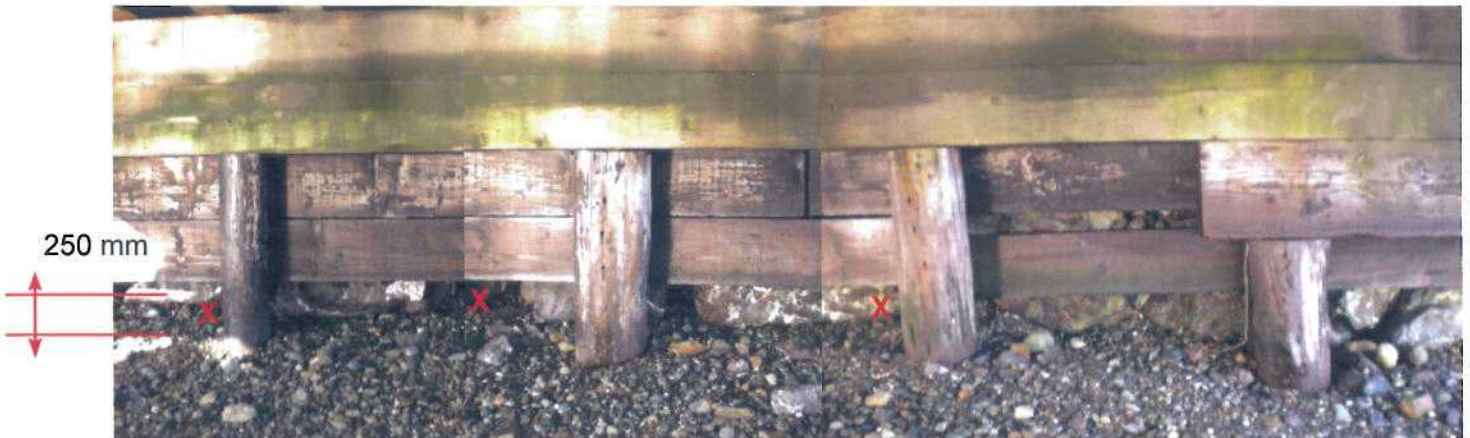
P7 - North Abutment face. Shows beach gravel erosion to 250 mm below the lowest 4x12 boards, exposing large rip-rap behind with washout of the finer backfill material causing voids. Note: 4x12 board on right side has dropped approximately 130 mm (it was probably placed on the old beach level and is not fastened to the back of the piles).
