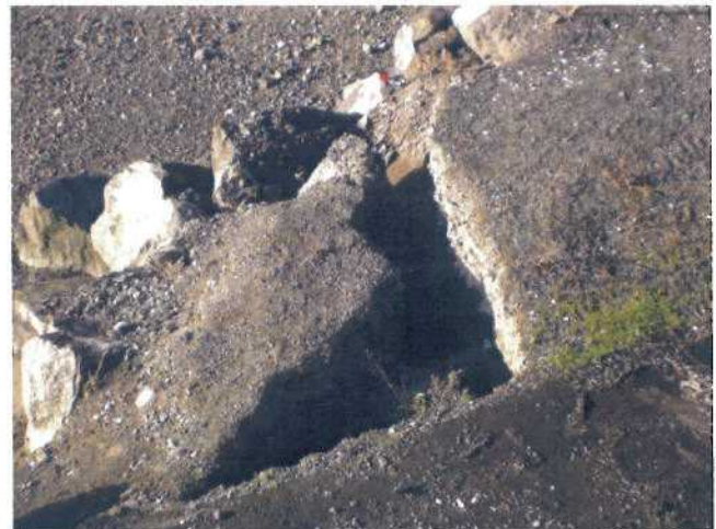
P4 - North Abutment Approach, Lagoon side, side view. Shows cleft caused by loss of backfill fines into voids between rip-rap blocks.
