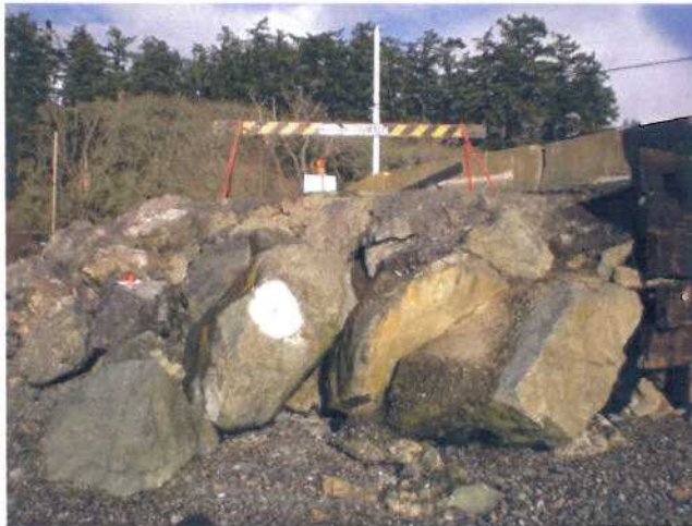
P1 - North Abutment Approach, Lagoon side. Beach gravel erosion (lowering) causing movement of rip-rap.
