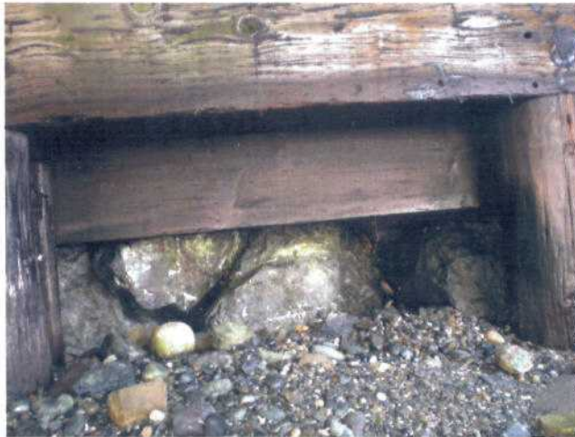
P12 - Close-up detail of P10 washout. Void behind penetrated to distance of 1300 mm. Beach gravel 300 mm below bottom of lowest board.
