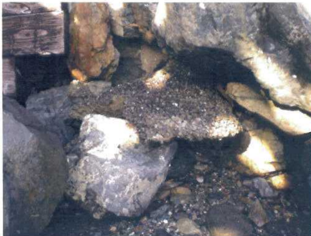
P15 - Close-up view of lower part of P14. Shows rock with concrete layer above it. This indicates old beach level and extent of gravel erosion that has occurred from underneath.
