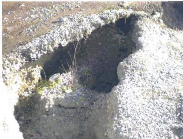
P3 - North Abutment Approach, Lagoon side. Cleft in backfill fines at edge of pathway asphalt. Cleft approximately 400 mm wide.
