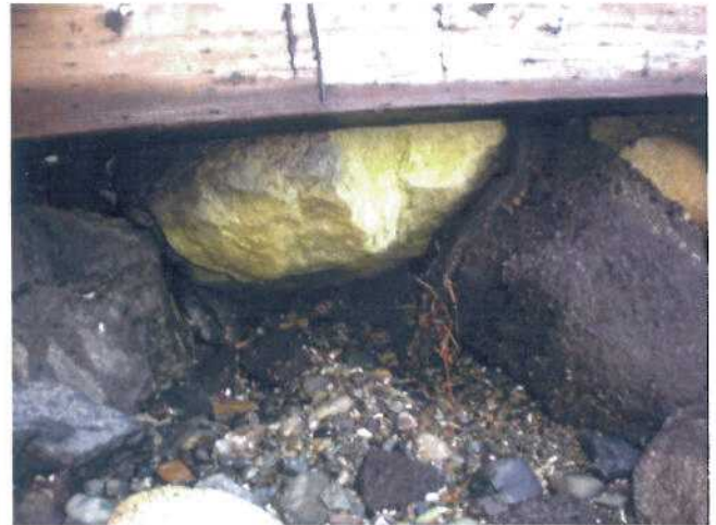
P13 - Close-up detail of P11 washout. Void behind penetrated to distance of 1000 mm. Beach gravel 430 mm below bottom of lowest board.
