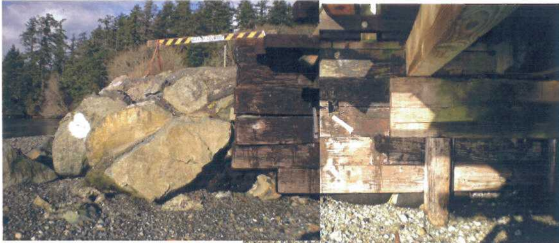
P5 - North Abutment, Lagoon side. Showing (on left) large rip-rap and timber 4x12 cantilevering from behind piled abutment. Beach level has been eroded away causing rip-rap to move and promoting erosion of fines into voids.
