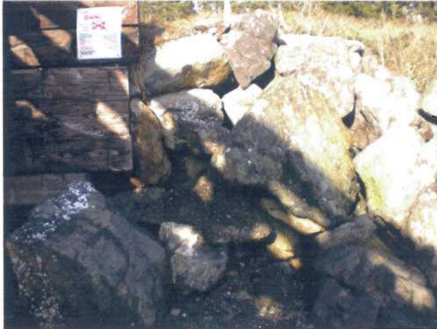
P14 - North Abutment - seaward side. General view of rip-rap beyond edge of wing wall boards.
