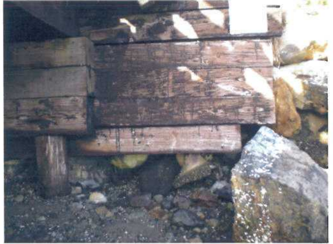
P11 - North Abutment - seaward side 'wing wall' planking cantilevering from behind pile line.
