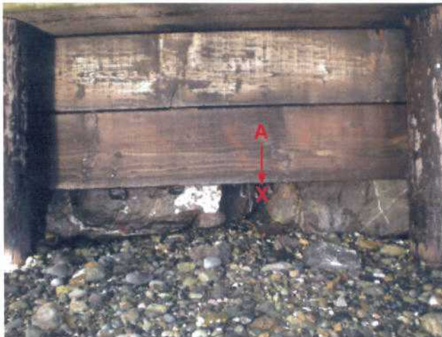
P8 - North Abutment face. Close up at base of boards. Point A was penetrated by a steel tape (into voids) 1300 mm. Voids also extend up behind the boards towards the roadway surface.
