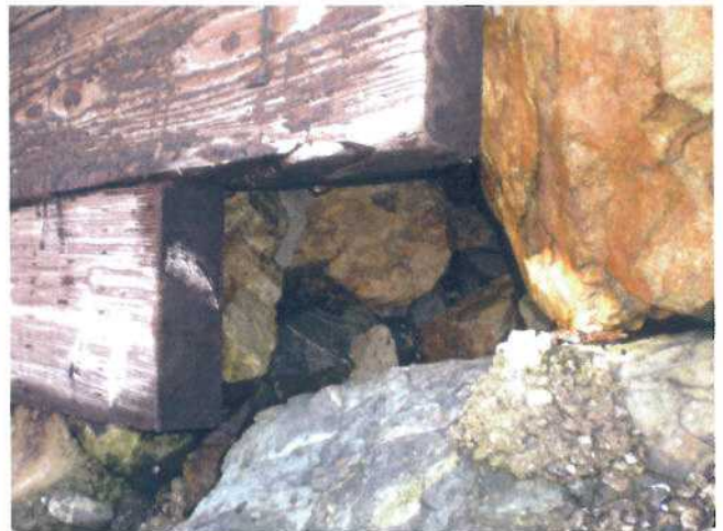
P16 - Close-up view of rocks behind wing wall showing absence of fine material due to washout.
