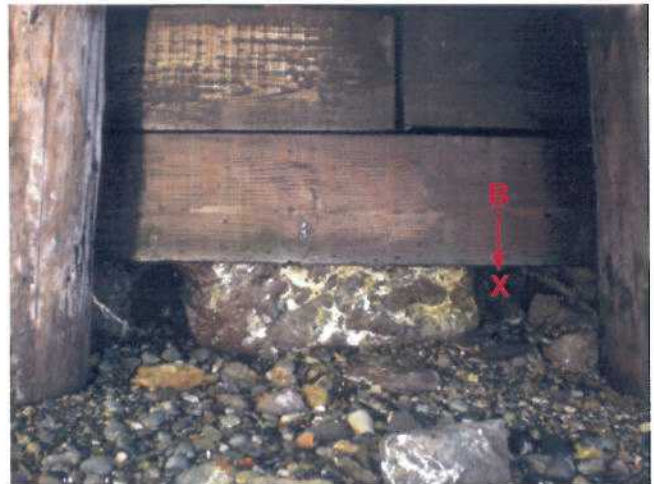
P9 - North Abutment face. Close up at base of boards. Point B was penetrated by a steel tape (into voids) 1900 mm. Voids also extend up behind the boards towards the roadway surface.
