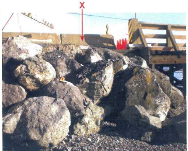
P2 - North Abutment Approach, Lagoon side, side view. 'X' shows cleft caused by loss of backfill fines into voids between rip-rap blocks.
