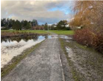
Existing: Trail washout due to seasonal flooding
