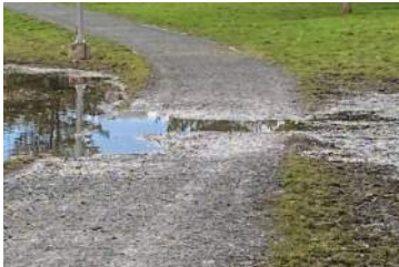
Existing: Trail washout due to seasonal flooding
