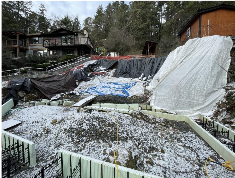
Photo 4. View looking west. Gravel has been placed for the foundation walls. There is no evidence of erosion or impacts being made to the surrounding environment. January 16,2024
