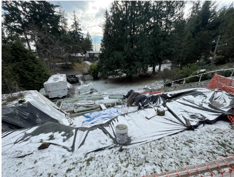
Photo 2. View looking east at the excavation of the proposed pool and structure. January 16,2024
