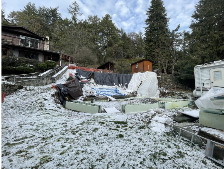
Photo 1. View looking west at the excavation of the proposed pool and structure. January 16,2024
